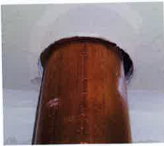
Copper Medical Gas Lines
