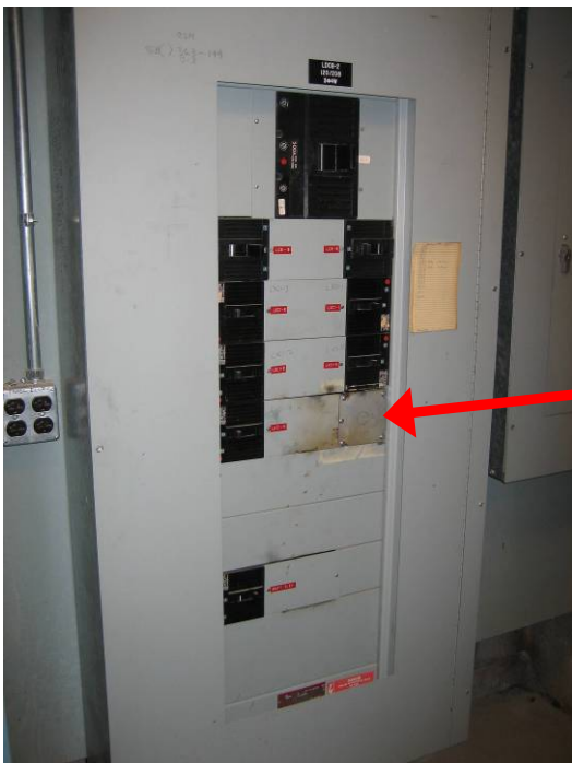
Electrical panel involved in incident
