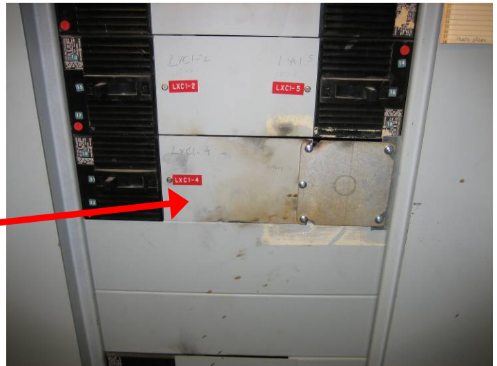
Close up view of installed cover. Right side of this cover contacted live parts during installation resulting in an arc flash.
