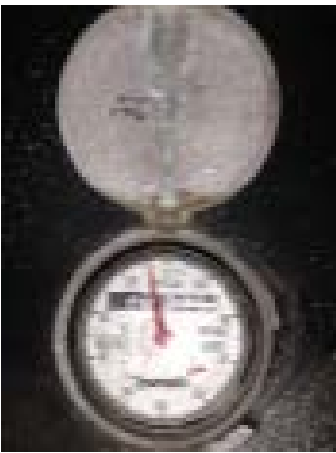
CE West Exterior Meter
