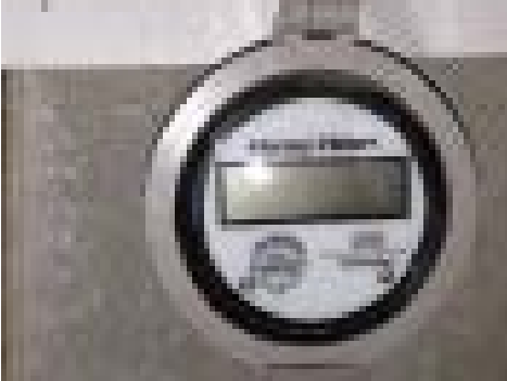
CE East Exterior Meter
